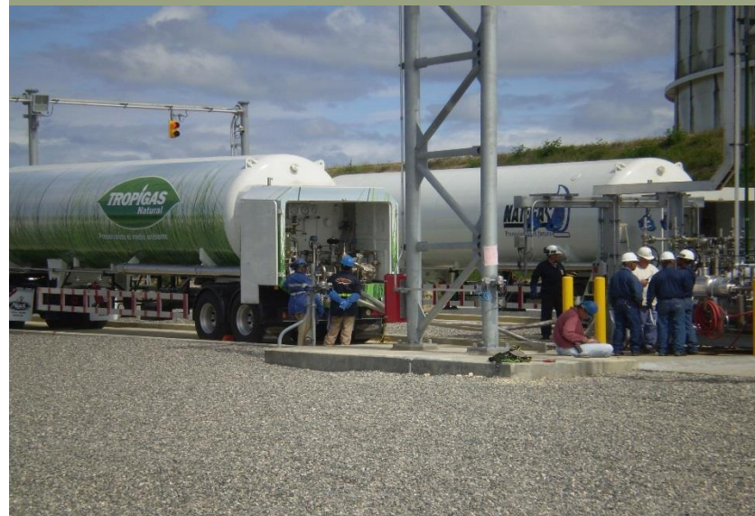
Two bay loading system at AES, Dominican Republic
