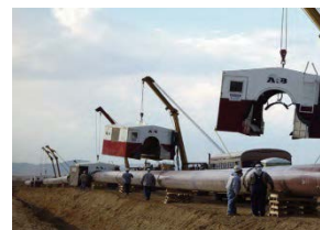
Kern River Pipeline
