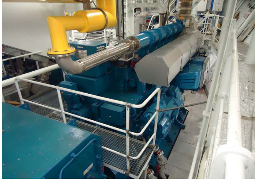
Wärtsilä dual fuel 6L34DF generator set onboard the PSV Viking Princess with double-walled gas supply line in yellow
